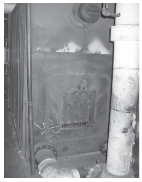
After 50 years of service at Beecher Road School, this boiler and its tandem partner (already scrapped) have been replaced.
