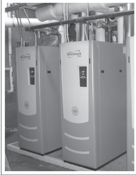
Three new high efficiency replacement gas boilers were commissioned for service in January.
