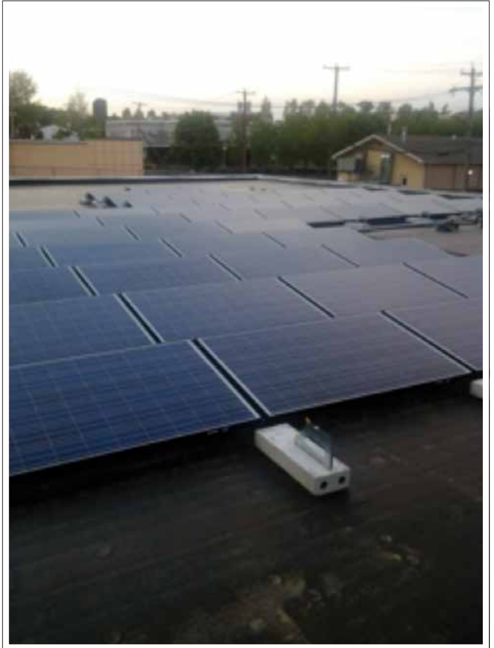
Solar panels on the roof of the Amity Teen Center
