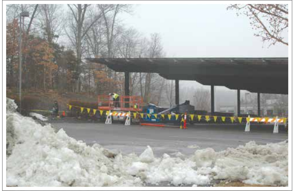
Installers of the solar car port at the JCC had to work through some harsh winter months to get the canopies up. A ribbon cutting July 16 celebrated the successful completion of the project.
