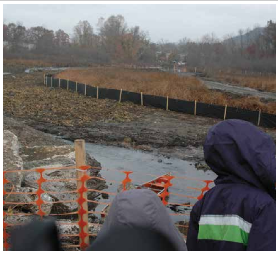
The West River will be diverted above the remnant of the dam to allow the riverbed to be restored and silt removed.
